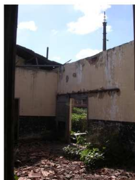
interior - telhado desabado
