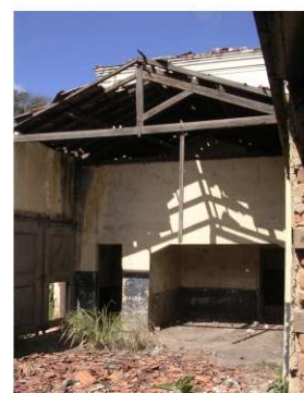
interior - telhado desabado
